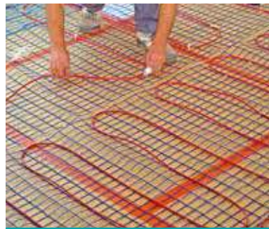
Heating cables connection.
